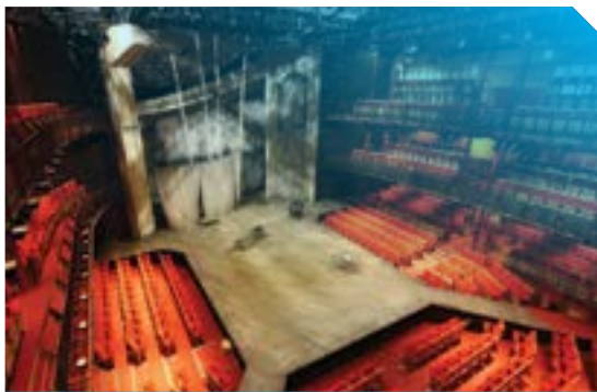
Ampetronic Hearing Loop installed in Royal Shakespeare Courtyard Theatre, Stratford upon Avon, UK
